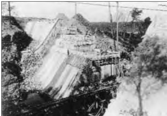
Lift by lift, the dam began to rise. With a gaping hole in the middle to accommodate the railroad tracks and to pass storm water, the two ends were constructed . . . slim at the far end, but fat in the middle to ensure stability. (November 2, 1914)
