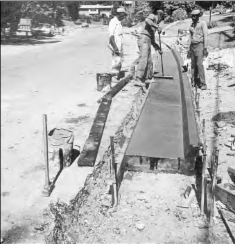
Responding to a WID engineering design by Ken Young of GKY & Associates, VDOT constructed a curb and gutter system to replace roadside ditches at the intersection of Nevius Street and Beachway Drive to improve safety of a school pedestrian crossing.
