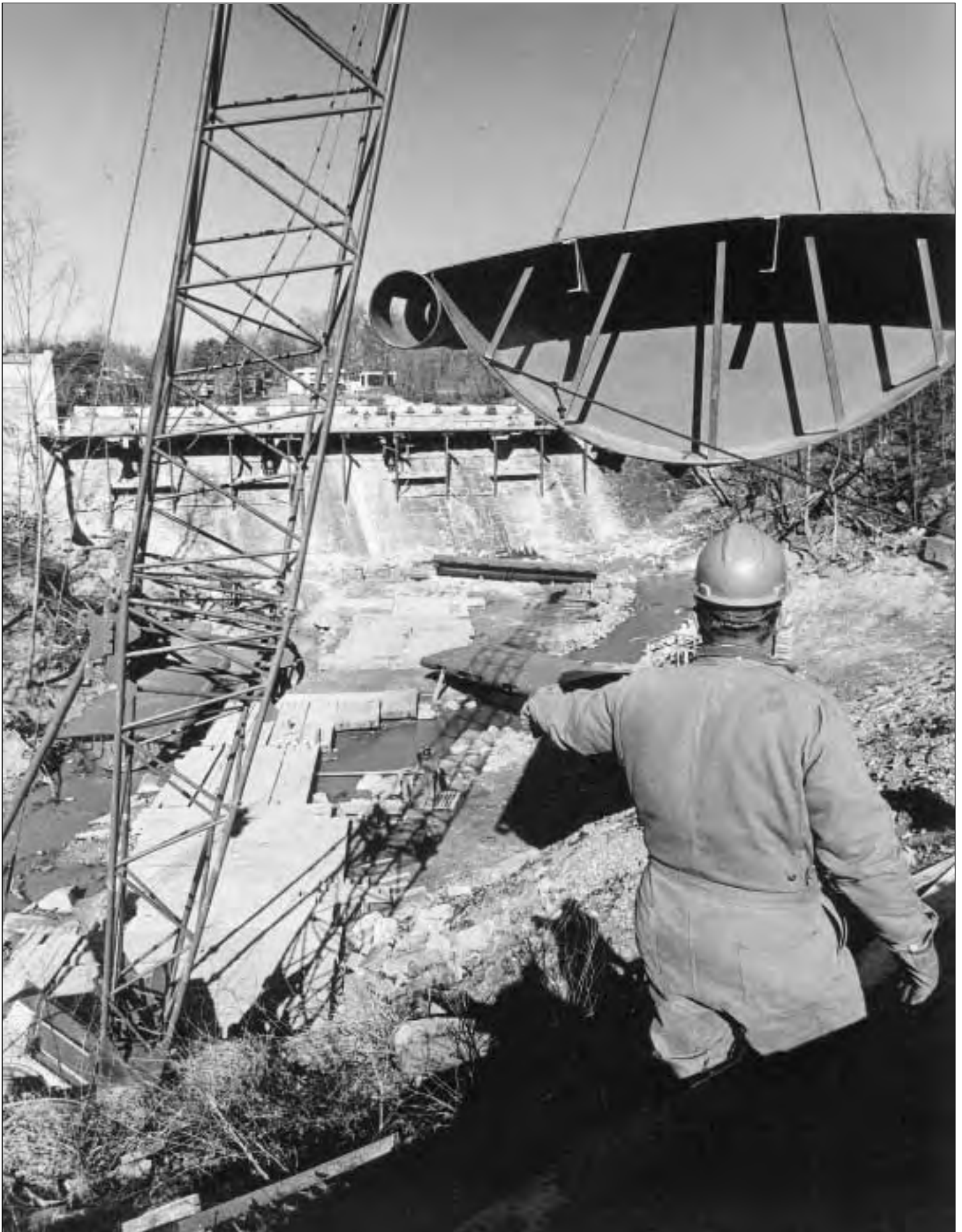
One section of the new, 150-foot Bascule Gate being lifted onto the Barcroft dam by crane. ( February 28, 1974 )
