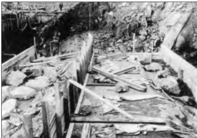
Engineers have quibbled whether the Barcroft Dam is a true Cyclopean Masonry structure. These rocks laid on top of concrete waiting for the next pour verify that it indeed does have a Cyclopean mix of rock and concrete. (November 30, 1913)
