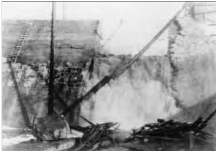
Before completion, Piedmont Construction Company went broke. This freshet pouring through the incomplected dam illustrates its problems. Somehow, we know not how, the Alexandria Water Company managed to finish construction. (About 1915)
